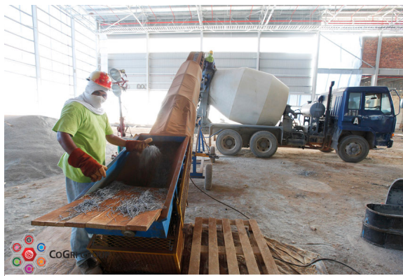
Fibre Integration At Site
